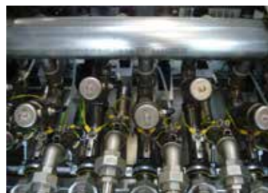
Water cooling systems
