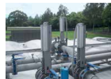
Controlled sluice gate for flowrate of return sludge at a wastewater treatment plant
