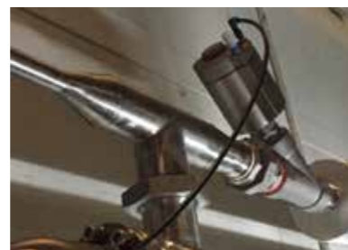
Shut-off control for glycol used in food production
