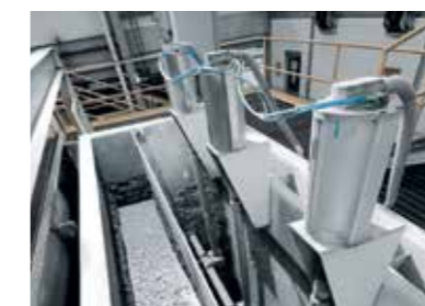
Control of dart valve for level regulation in mineral processing
